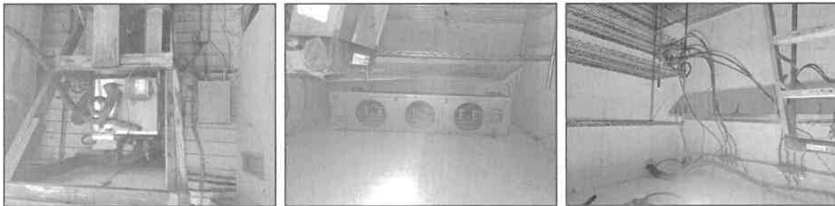
8.5 Item 1 (Picture) 8.5 Item 2 (Picture) 8.5 Item 3 (Picture) The walk in refrigerator was not inspected or tested. Recommend further evaluation.
